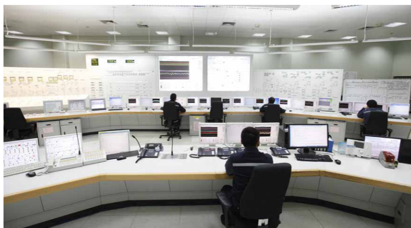
The main control room of Jiangsu Nuclear Power Unit 2
