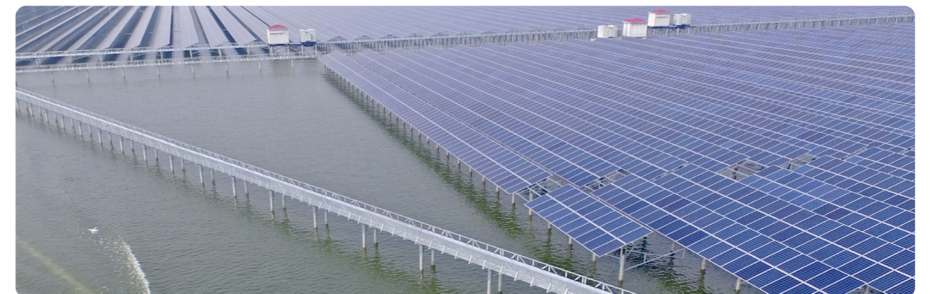
China Rich Energy Corporation Limited fishery-solar hybrid project in Nandagang, Cangzhou
