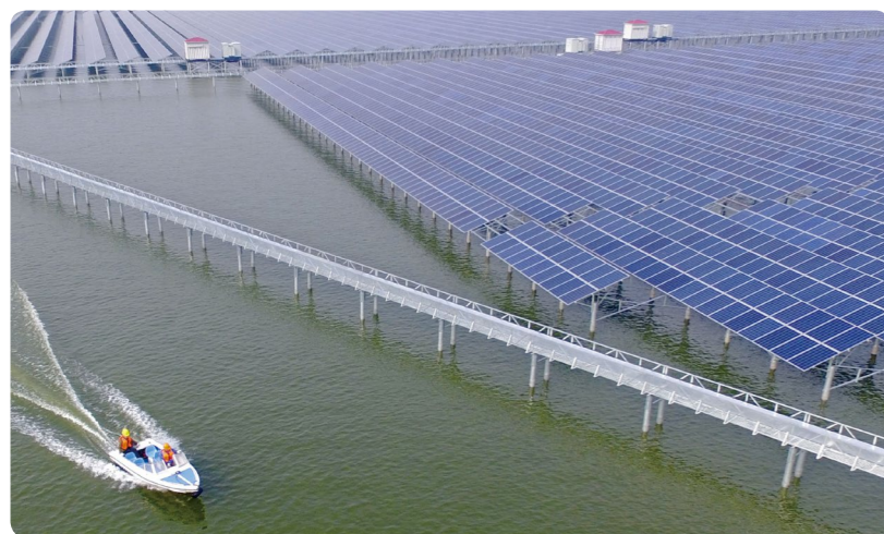
China Rich Energy Corporation Limiteds fishery-solar hybrid project in Nandagang, Cangzhou
