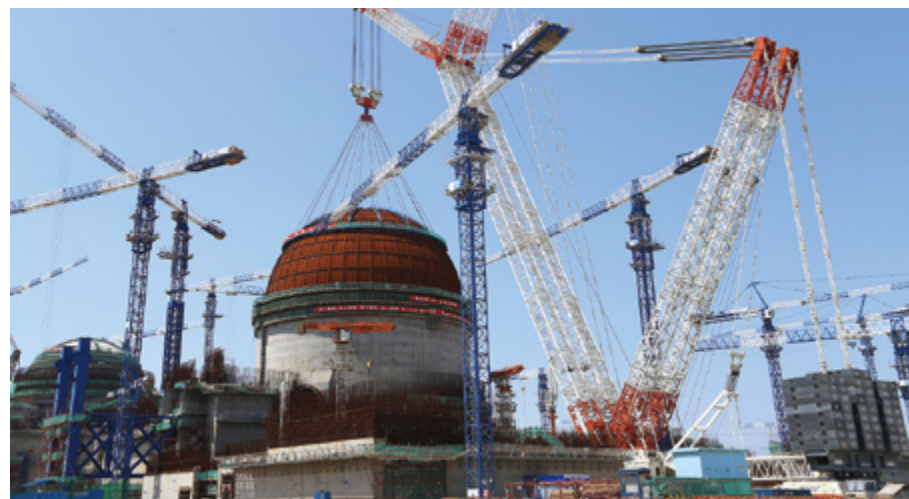
Successful hoisting of the dome of No.5 unit of Fuqing Nuclear Power, the world's first "HPR1000" demonstration project "Hualong No.1"
