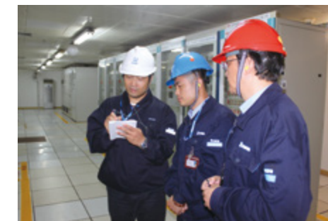
A follow-up visit to Qinshan Nuclear Power No.2 Plant after WANO peer review
